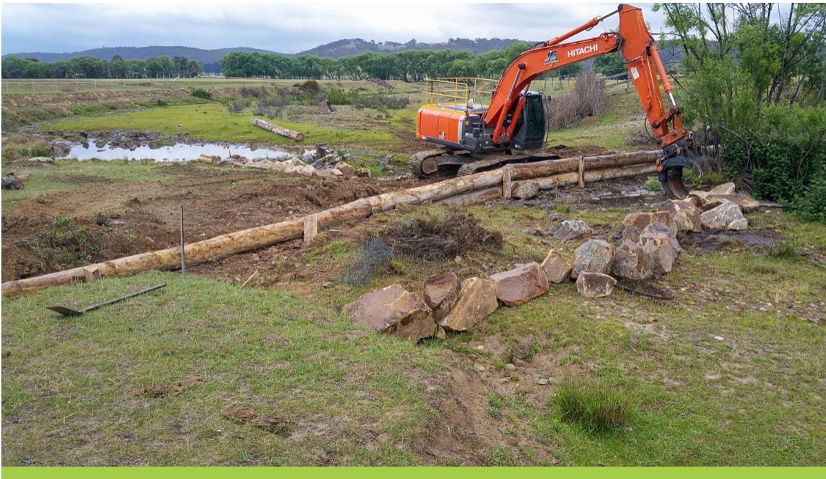
[IMAGE: During installation of a ‘landscape rehydration infrastructure’ at Westview Farm in 2018.]
